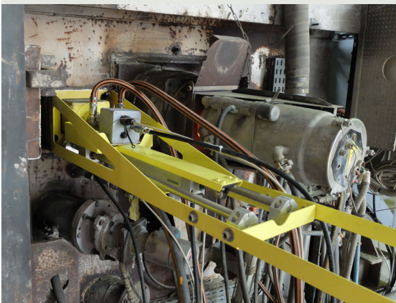
→ Pyroscan installed close to the kiln burner
